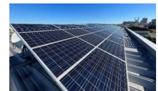
Installed solar power at Osaka-Minami office(2013)
